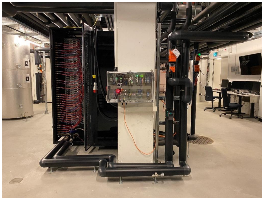
Figure 5 Picture of the liquid-cooled [23] servers integrated into the NEST building [22].
